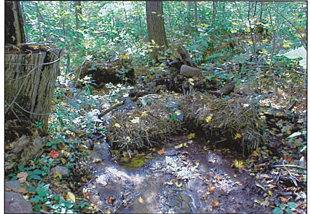
When placed in smaller creeks and drainages, hay bales can provide an effective temporary sediment trap downstream from a stream crossing.
