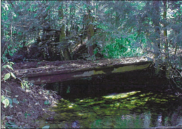
Temporary bridges provide an effective stream crossing for heavy equipment and helps protect and minimize disturbance to the streambed and banks.
